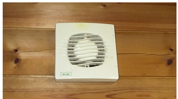
Extractor fan not working
